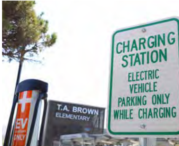
Electrical Vehicle Charging Station
