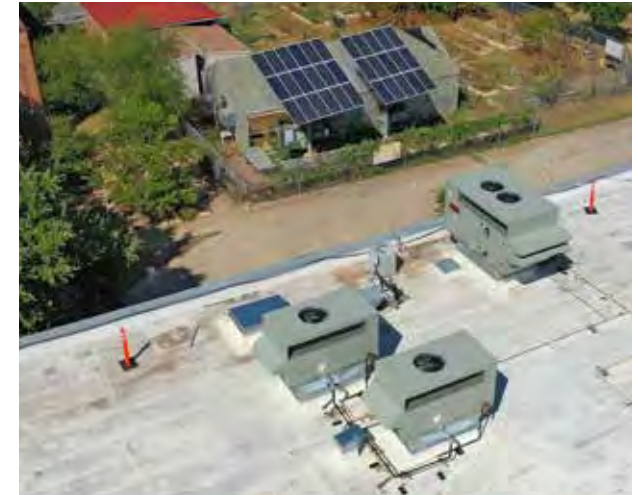
Solar and HVAC Systems
