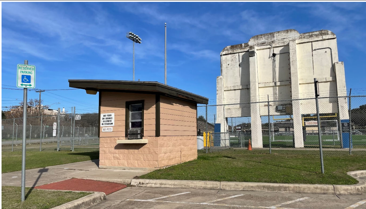
Ticket booth is in adequate condition but is small.
