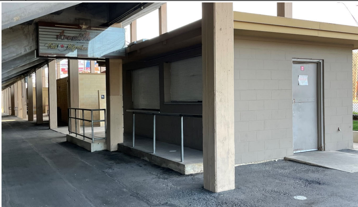
View of the concession stand exterior. Dated/ worn appearance and not ADA compliant.
