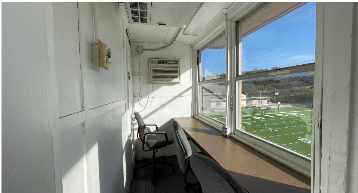
View of one of the press box spaces. Spaces are equipped with wall units. There is no elevator access to the press boxes, and the windows leak. The space does not accommodate the number of people who need to use it for events.
