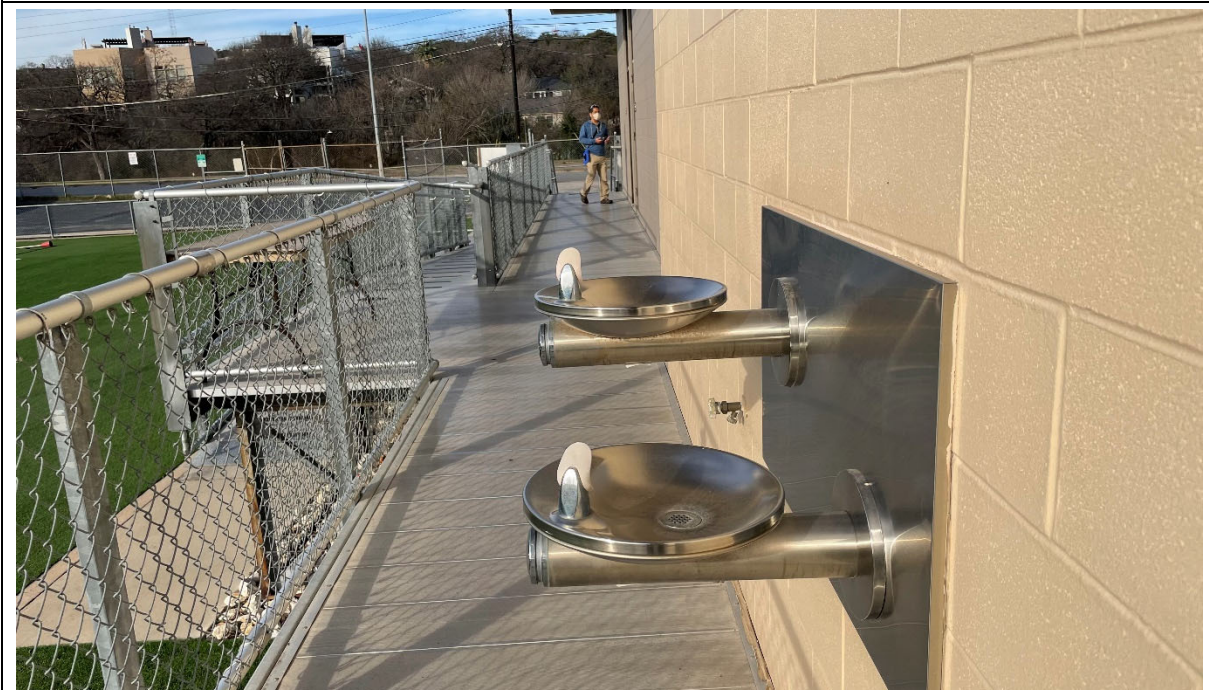
Drinking fountains protrude into circulation path therefore they are not ADA compliant.
