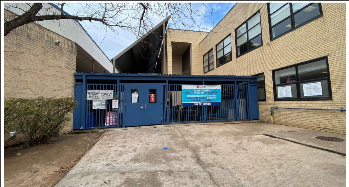
Main Entrance: Lack of signage and wayfinding make it difficult to understand this is the main entrance. Additional signage has been posted since this photo was taken; however, additional signage is still needed.
