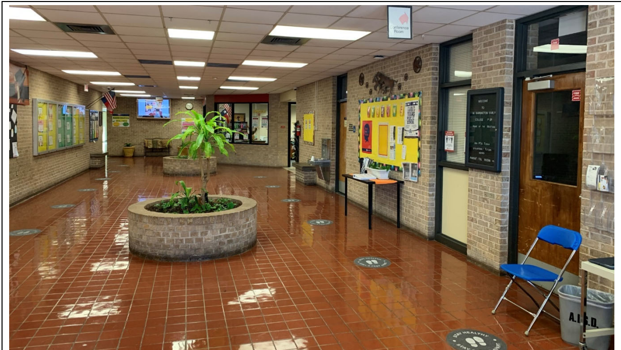
Main entry area is spacious and feels welcoming with displays and planters. The main entry does not have a secure vestibule and is far from reception at the end of the lobby.
