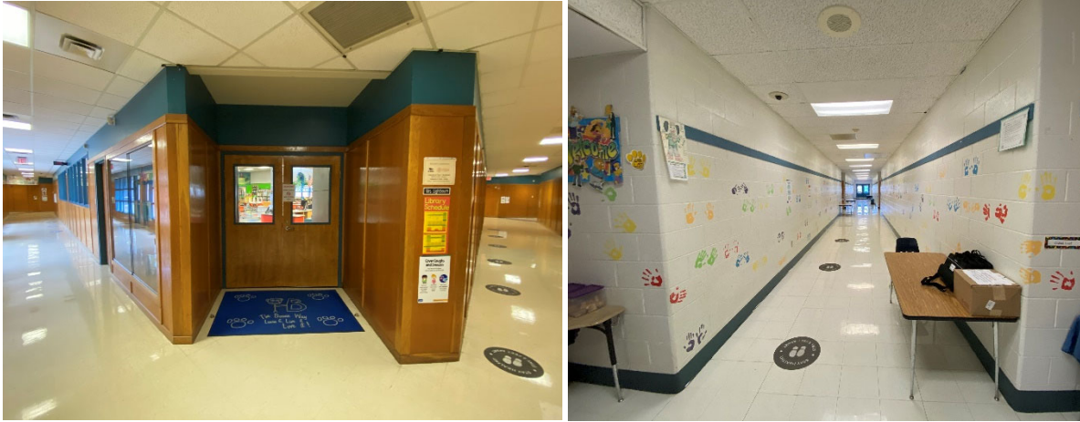
Some corridors have updated finishes. Some have dated wood paneling. There is limited visibility from studios into corridors in some areas of the building.
