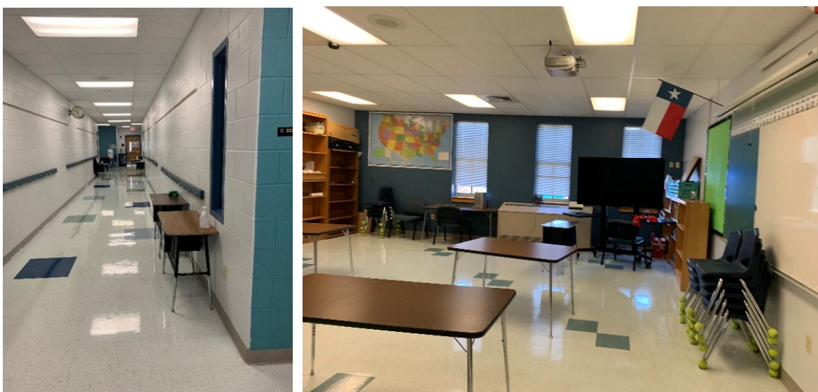
Academic Wing: Limited visibility between studios and corridors exists (left); furniture in the studios is outdated and difficult to reconfigure (right).
