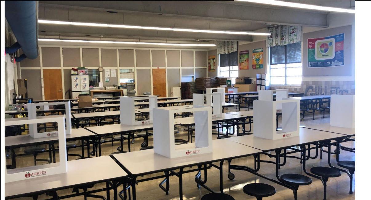
Cafeteria and kitchen are very undersized. Kitchen is 850 square feet and requires exterior freezer/coolers. Stage within cafeteria is not accessible.
