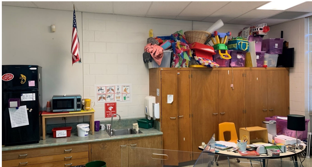
Casework storage is dated and insufficient throughout the school.
