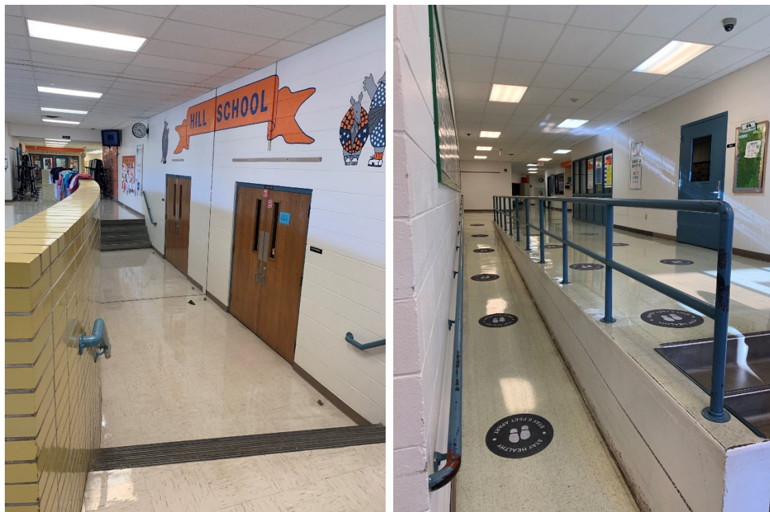
Steps to cafeteria and gym along main corridor. Accessible ramp is on side hallway.
