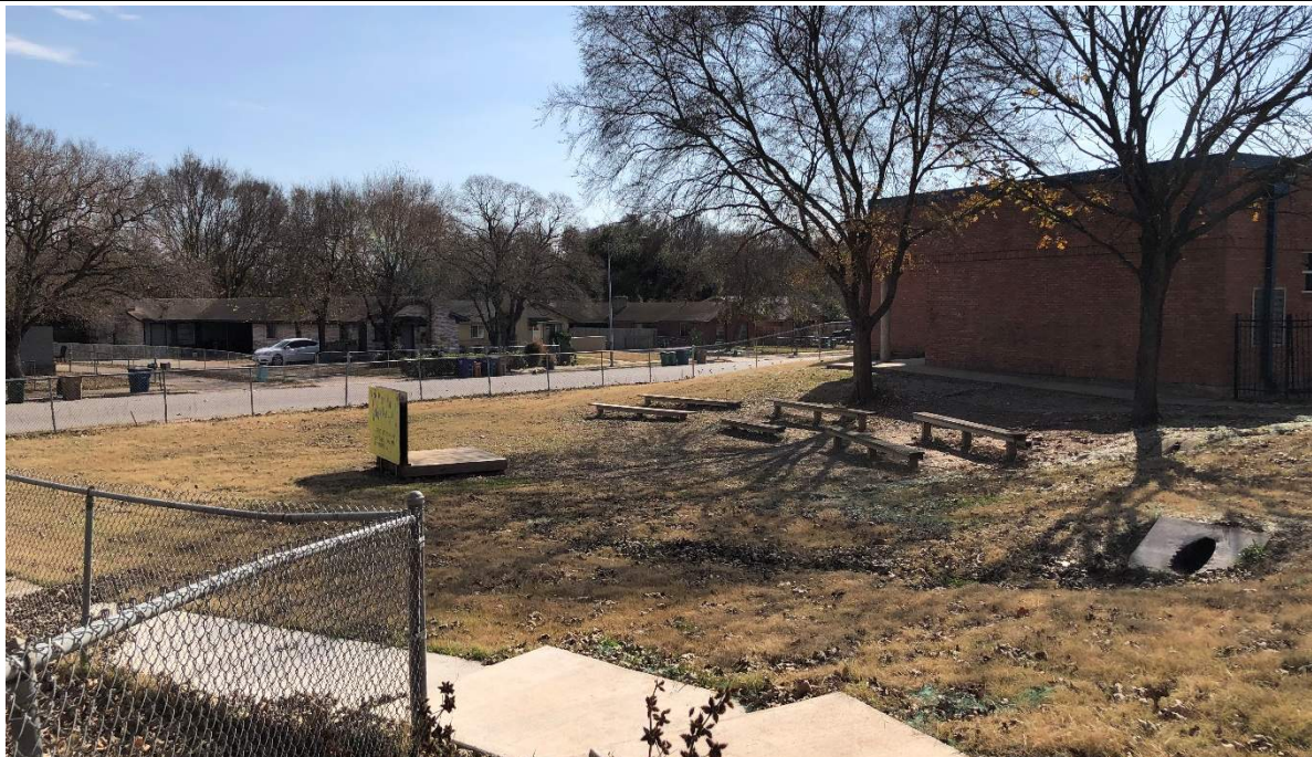
Main outdoor learning space with benches and platform. Some raised garden beds nearby but there is no water source or power outlets. The surface is not level due to erosion, which impacts accessibility.
