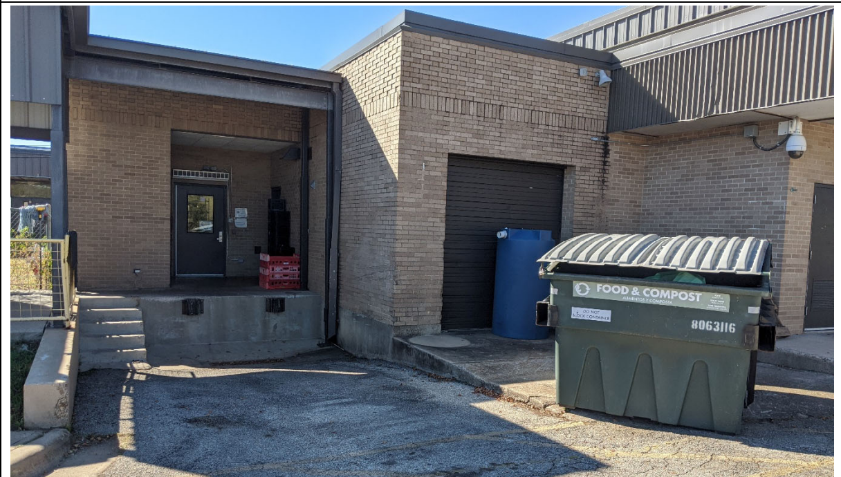
Loading dock but no accessible route for trash and compost.
