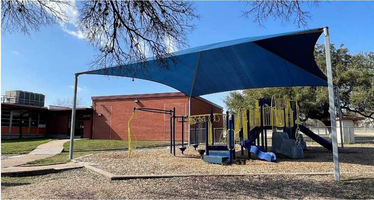
Outdoor Learning and Activity: Covered playscape is in good condition.
