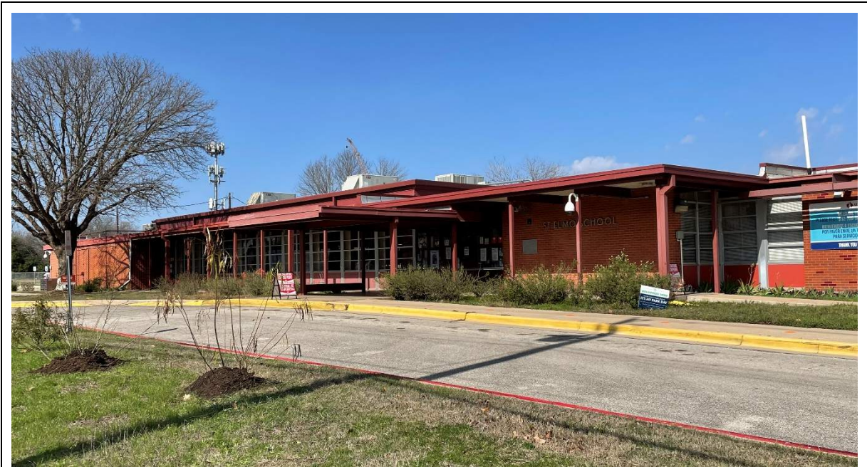
Exterior: Building exterior is in good condition considering the age of the school.
