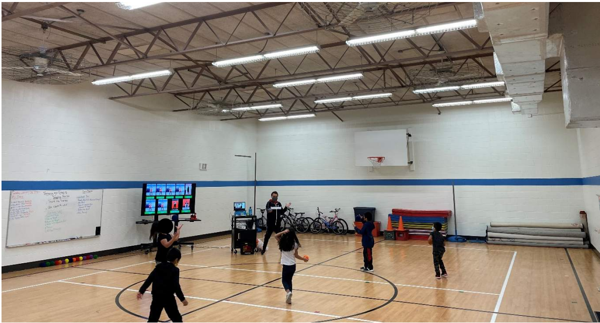
PE and Wellness: Gym does not meet size requirements in Ed Spec, with original hoops and no natural light. Support spaces are not adequate.
