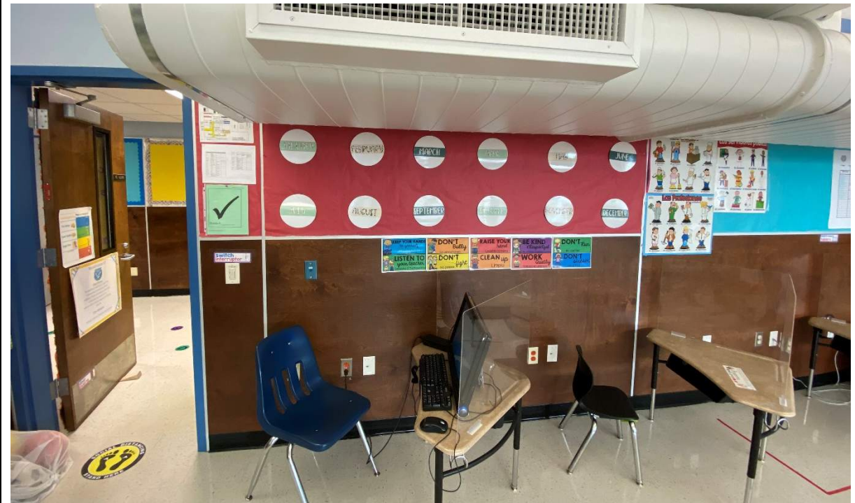
Relatively new HVAC duct hangs below acceptable head height in the older wing studios.
