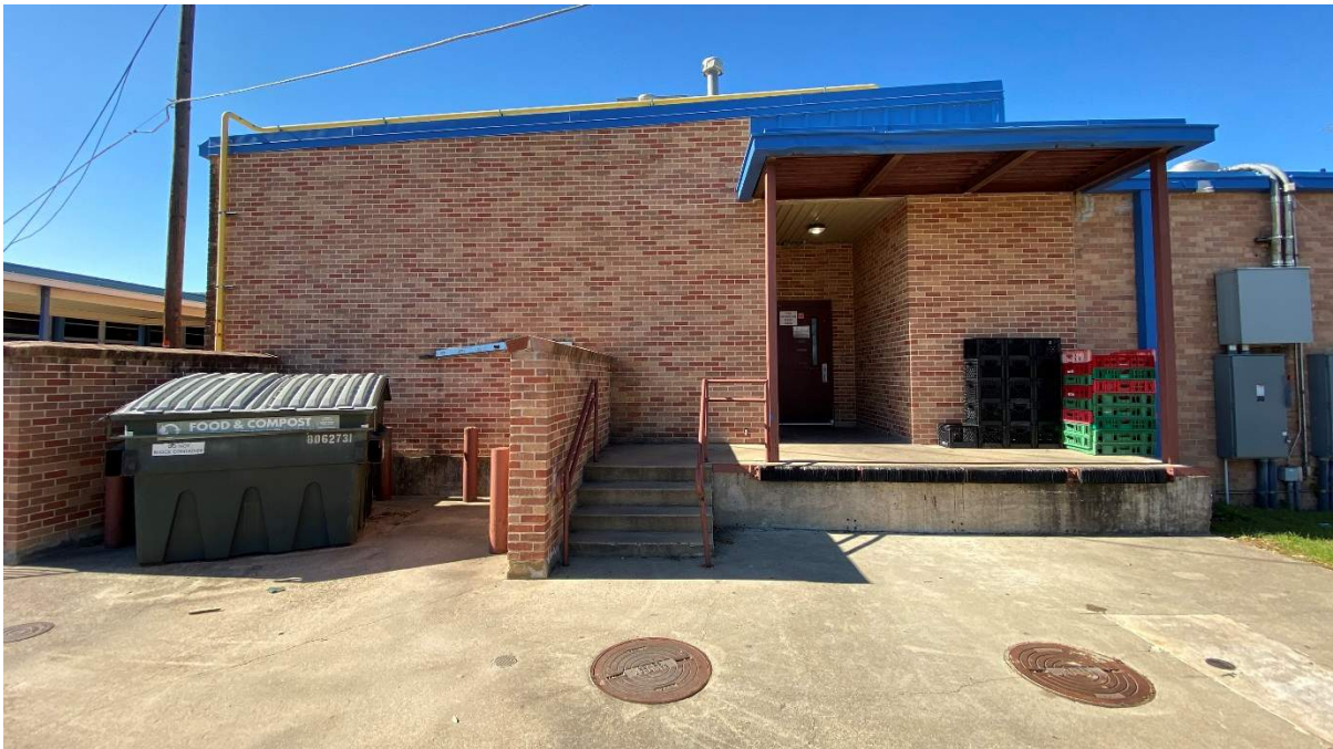
Dumpsters are not on accessible path. Compost is adjacent to exit; however, trash and recycling are 100+ feet away at the edge of the parking lot.
