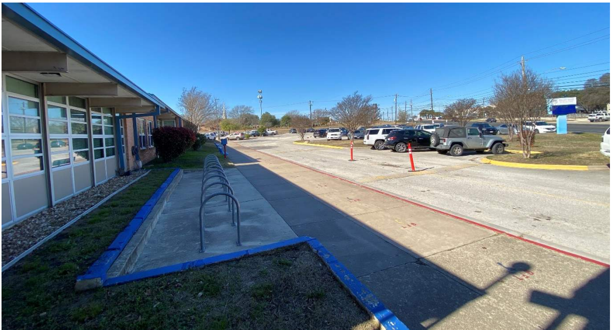
The drop-off at the main entrance doesn't have an overhang and does not separate bus traffic or pedestrian foot traffic through the parking lot.
