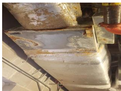
Classroom damaged variable air volume unit
