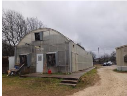
Corrosion on support beam of the greenhouse
