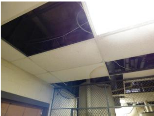
Missing acoustical ceiling tiles in the gym
