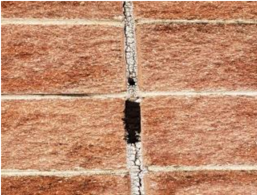
Cracked exterior brick
