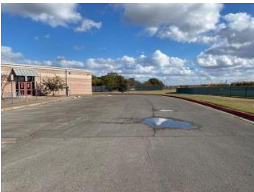
Asphalt pavement at end of life
