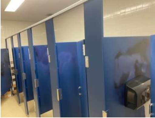
Restroom partitions at end of life
