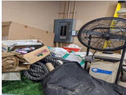
Obstructed electrical panel
