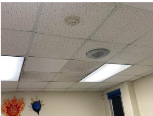
Acoustic ceiling and grid at end of life
