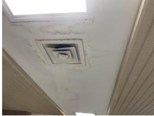
Stained cafeteria corridor ceiling
