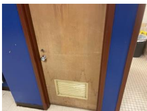
Water damage and bowing on wood doors
