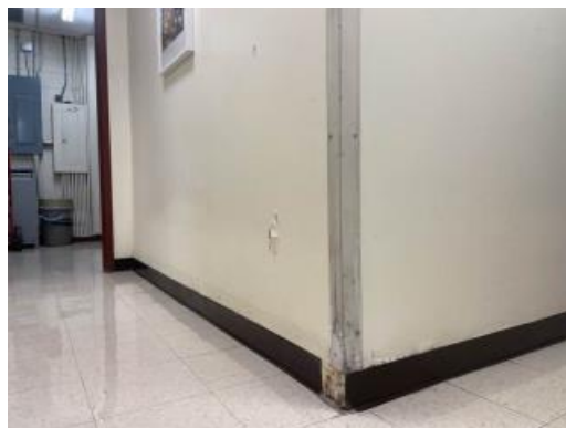
Administration wall finish damaged
