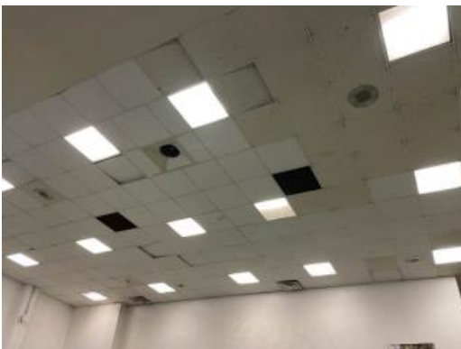
Acoustic ceiling tiles at end of life
