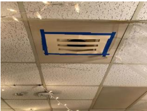
Cracked acoustical ceiling tile
