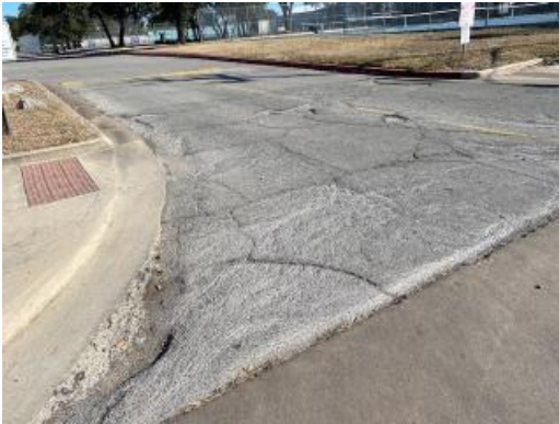
Damaged asphalt driveway
