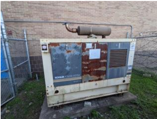
Corroded emergency generator
