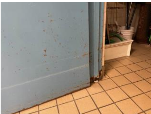
Steel door corrosion at bottom of door and frame
