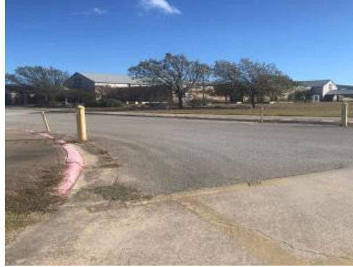
Cracked asphalt pavement
