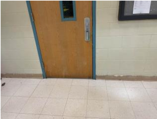
Sample Wood door delaminating at bottom and ends
