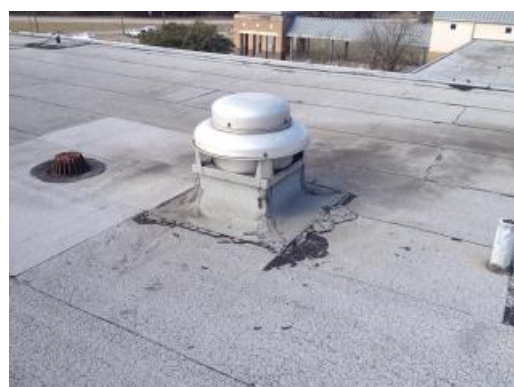
Damaged roof exhaust fan
