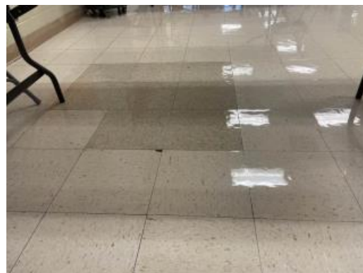
Vinyl composition tile flooring deficient
