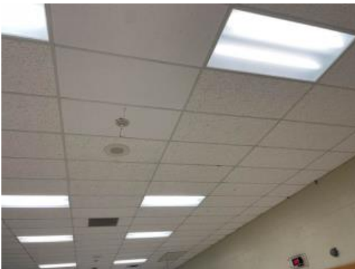
Sagging acoustic ceiling grid and tiles
