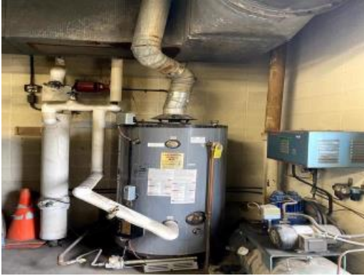
Rusted water heater piping
