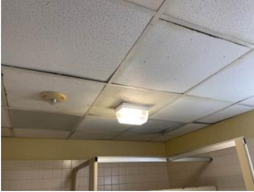
Restroom acoustic ceiling tiles past useful life
