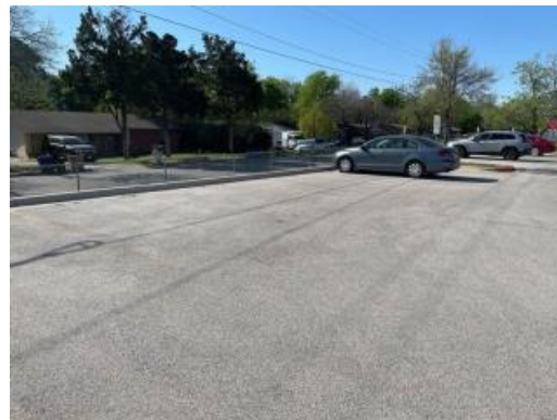
Parking lot missing striping
