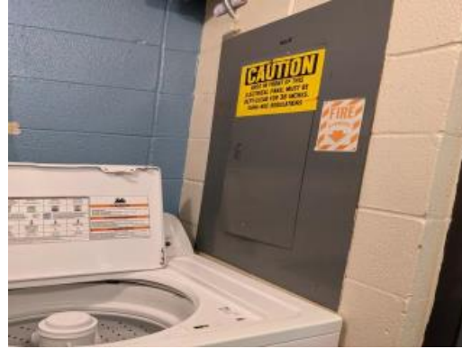
Obstructed electrical panel
