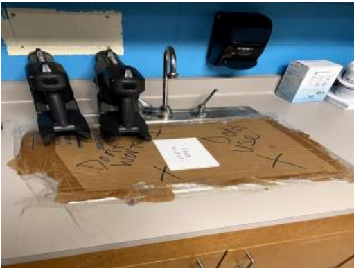
Classroom sink not working
