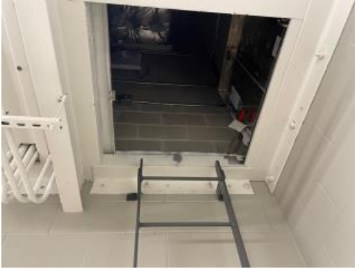
Ladder deficiency, cafeteria chair storage room.
