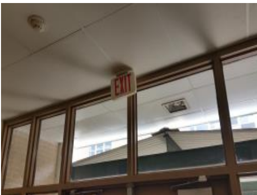
Burnt out exit light
