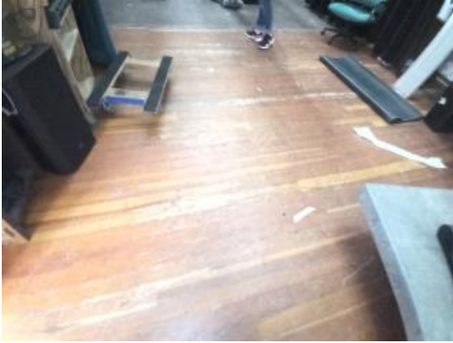
Well worn wood flooring
