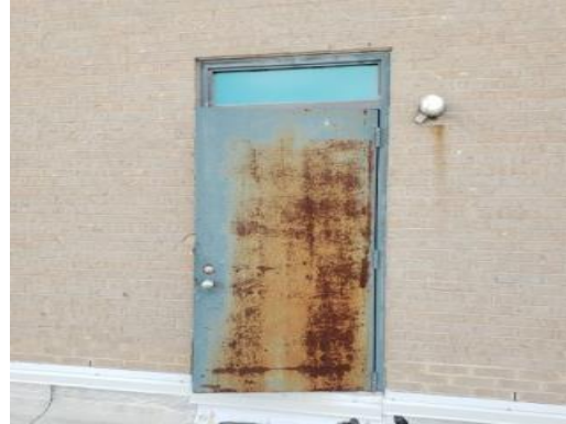
Rusted exterior door with faded paint
