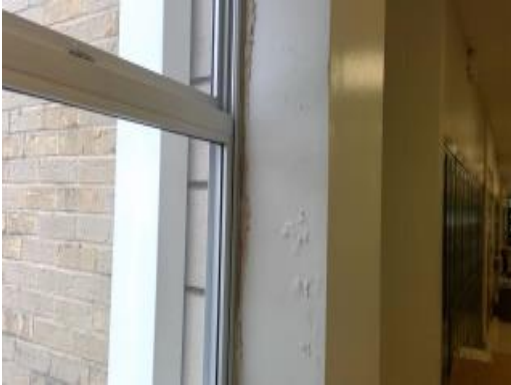
Water infiltration on interior wall
