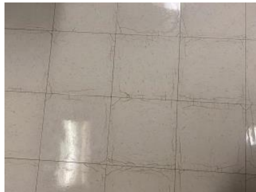
Cracked vinyl composition tile
