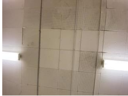
Aged ceiling tiles
