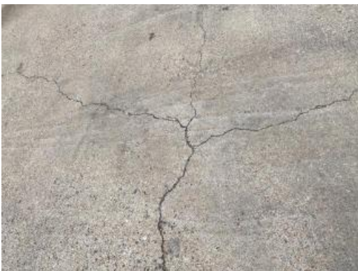
Cracked concrete pavement
