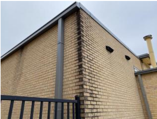
Stained brick wall
