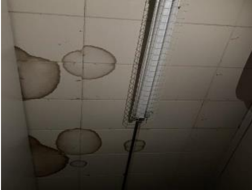
Stained ceiling tiles
