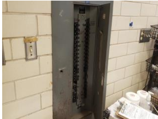
Electrical Panel Corroding
