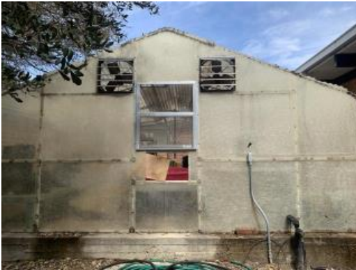
Green house needs painting and has broken window
