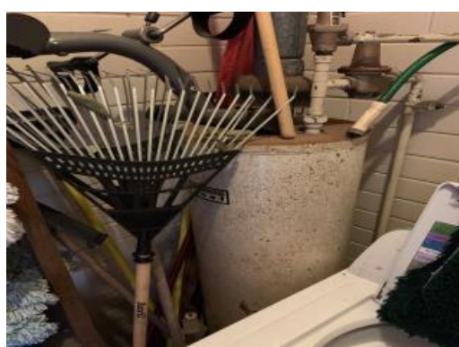
Water Heater Corroded
