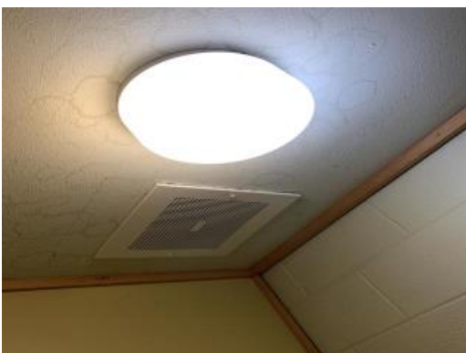
Stains on Ceiling
