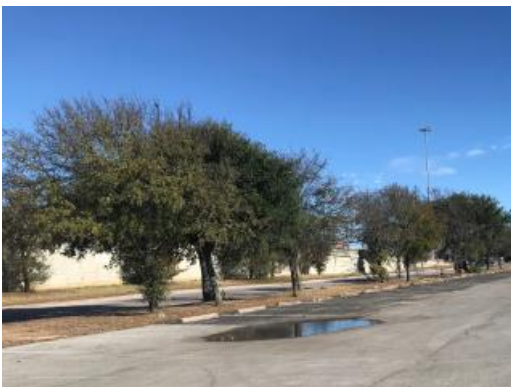
Potholes in parking lot
