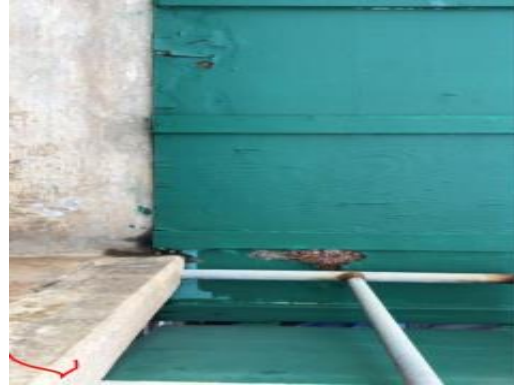
Damaged wood wall panels
