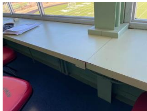
Fixed casework countertop delaminated
