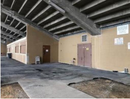
Well worn concrete slabs
