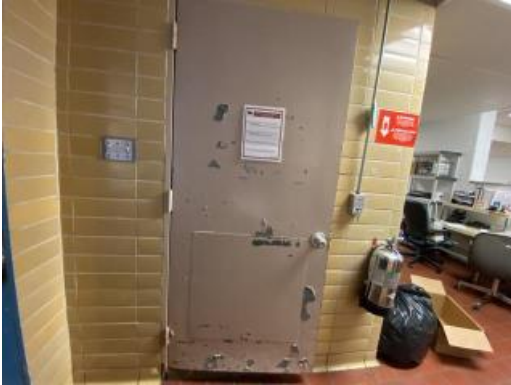
Damaged metal door
