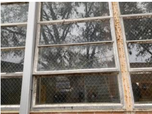
Aged exterior windows
