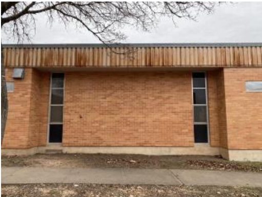
Rusted metal fascia
