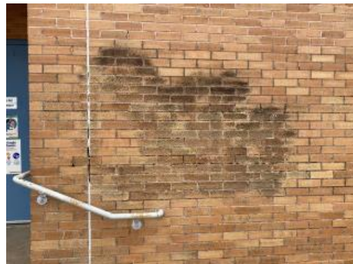
Stained exterior brick wall
