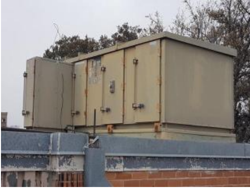
Corroded roof top unit
