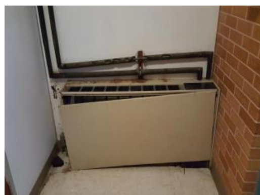
Damaged air conditioning unit
