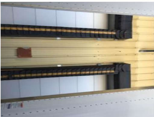
Damaged wall panels
