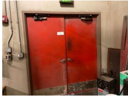
Steel doors are beyond their useful life
