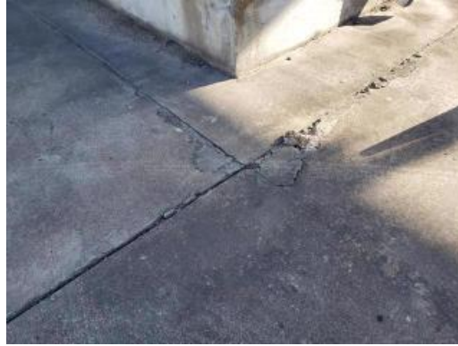
Cracked concrete pavement.
