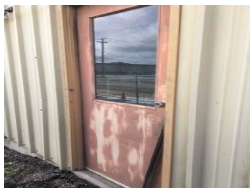
Steel doors are beyond useful life.
