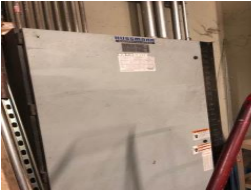
Hassmann panel inaccessible
