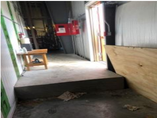
Steep drop off and is life threatening
