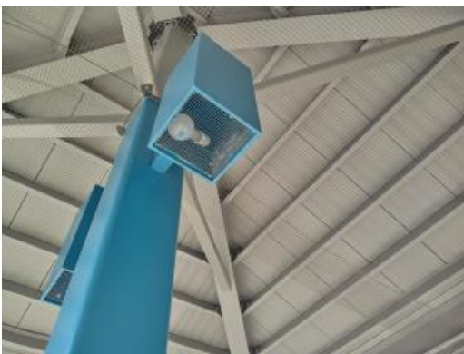
Exterior lighting system
