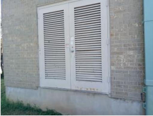
Exterior doorway is well worn
