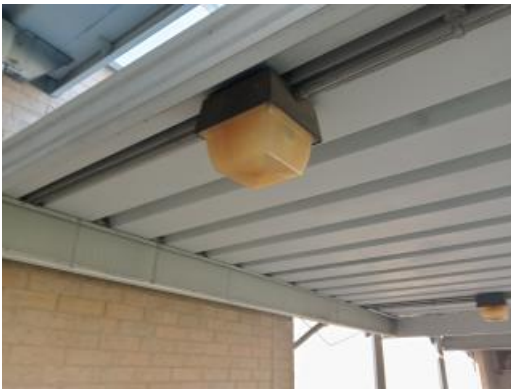
Light system is well used
