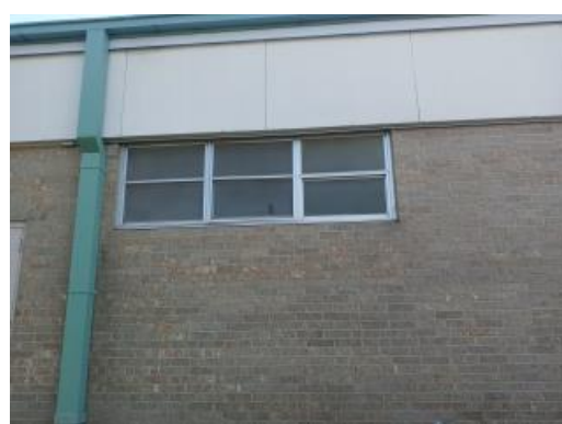
Exterior windows are beyond their useful life
