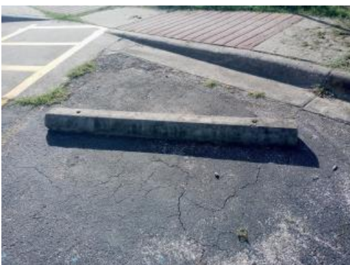
Paver marker is broken
