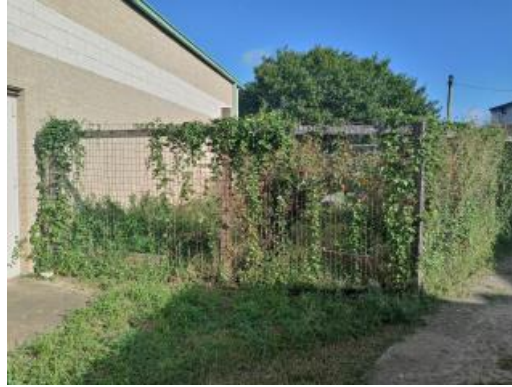
Fence is overgrown
