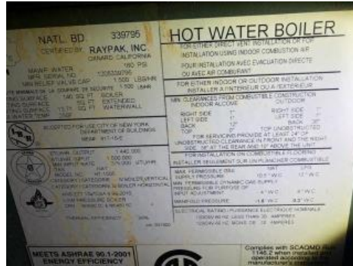
Hot water boiler beyond useful life
