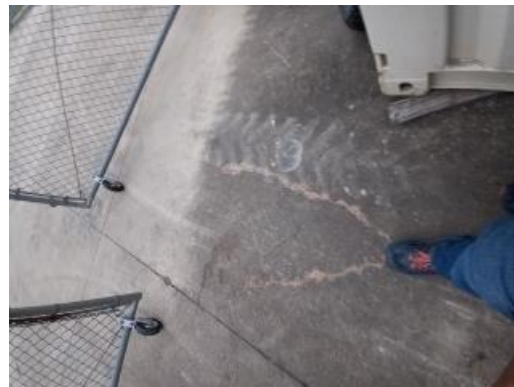
Concrete pavement is stained
