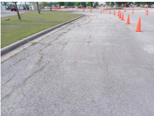
Asphalt pavement cracked and has vegetation growth
