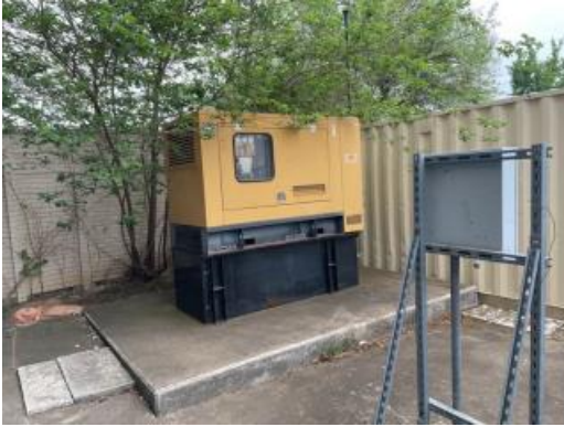
Generator is not functional
