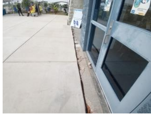
Exterior doors are worn
