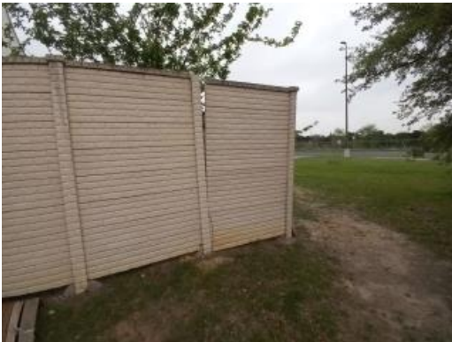
Exterior enclosure wall shows differential movement.
