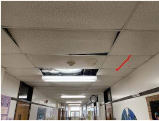
Damaged acoustical ceiling tile
