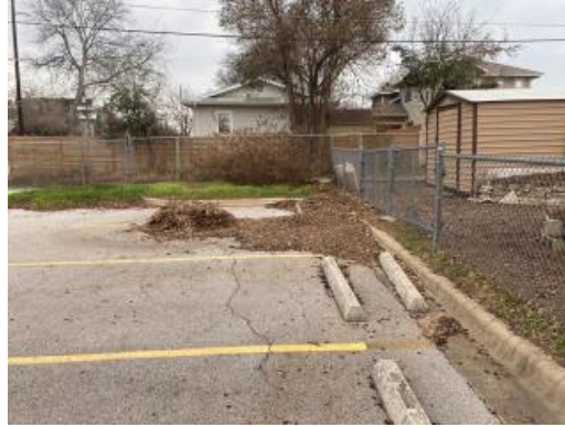
Asphalt paving damaged
