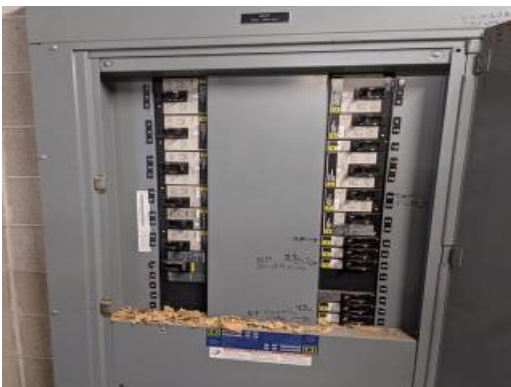
Electrical panel aged
