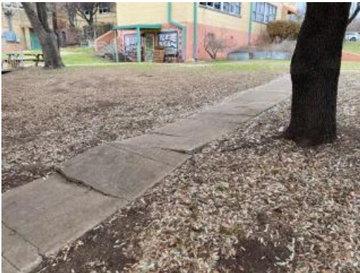
Damaged concrete sidewalks
