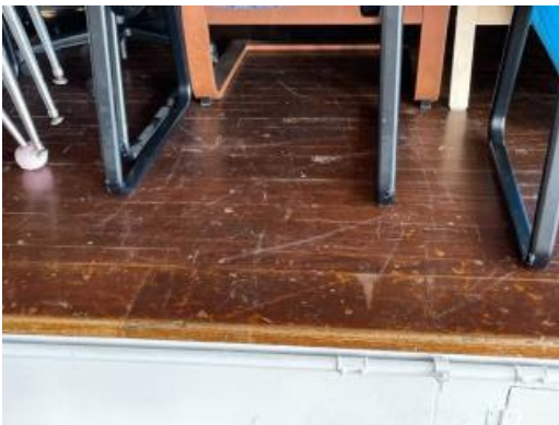
Stage wood flooring worn and torn
