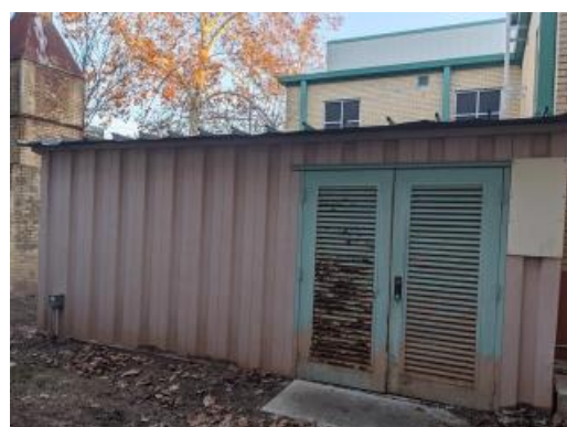
Exterior metal doors outdated
