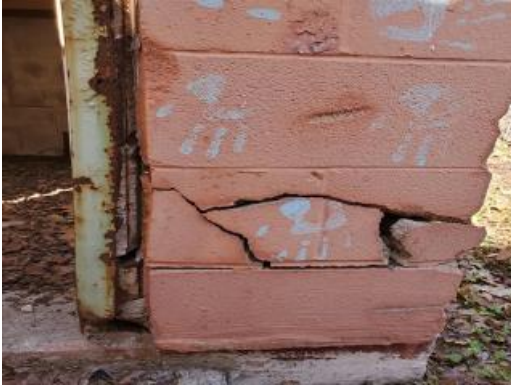
Damaged exterior concrete masonry unit
