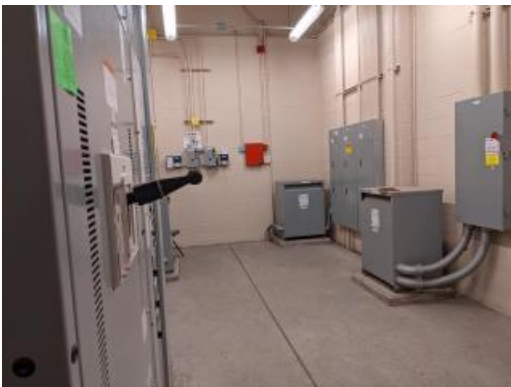
Electrical Panels and Transformers
