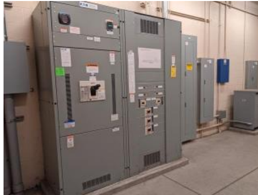
Main switch gear
