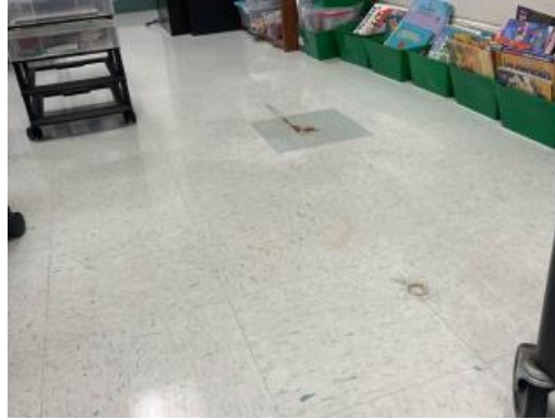
Stained and damaged classroom vinyl composition tile flooring
