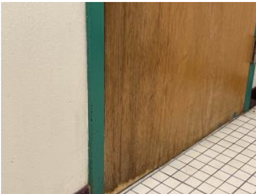
Damaged wood restroom door
