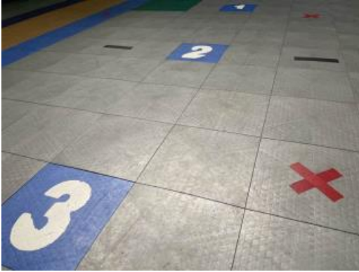
Corners are lifting and tiles have lost slip resistant texture on gym floor
