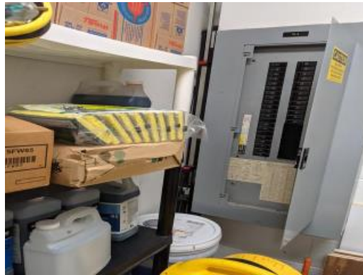
Obstructed electrical panel
