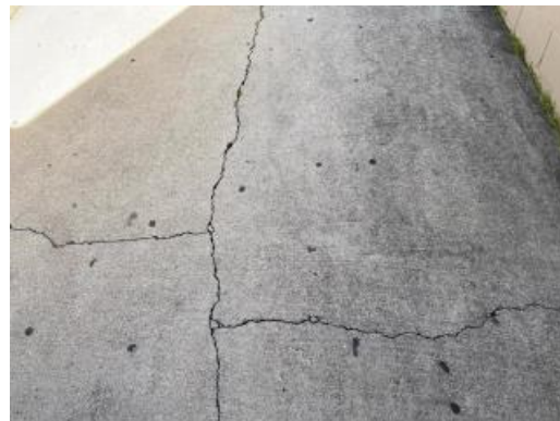
Asphalt pavement is cracked.
