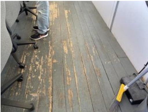
Wood floor is damaged, worn, and paint is flaking.
