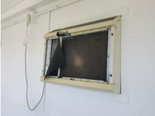
Window unit is beyond service life.
