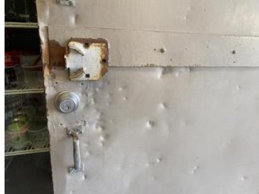
Metal door is rusted and damaged.
