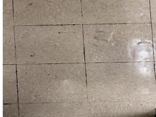
Vinyl composite tile flooring is damaged and worn.
