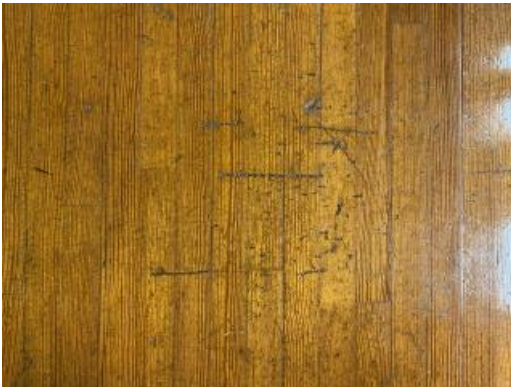
Scratched wood flooring
