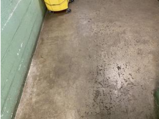
Concrete floor is damaged and stained.
