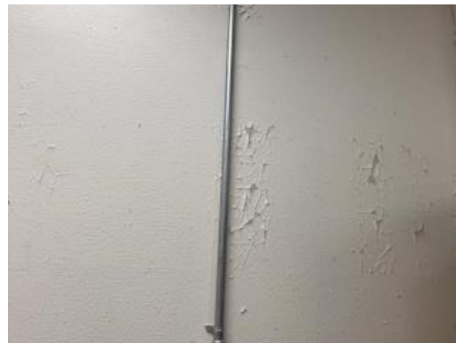
Cracked paint on interior walls.
