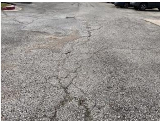
Asphalt is cracked and uneven.
