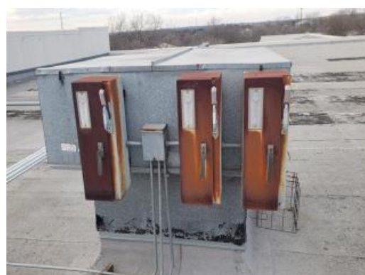
Aged roof top unit
