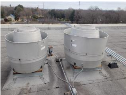
Vent roof fans are past life
