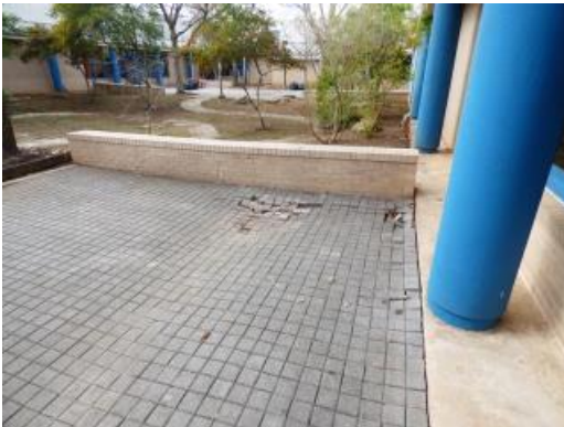
Pavers are damaged
