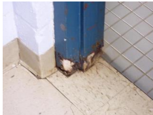
Door frames are corroded
