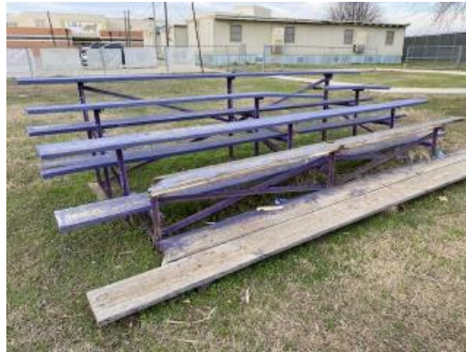
Bleachers are worn and broken
