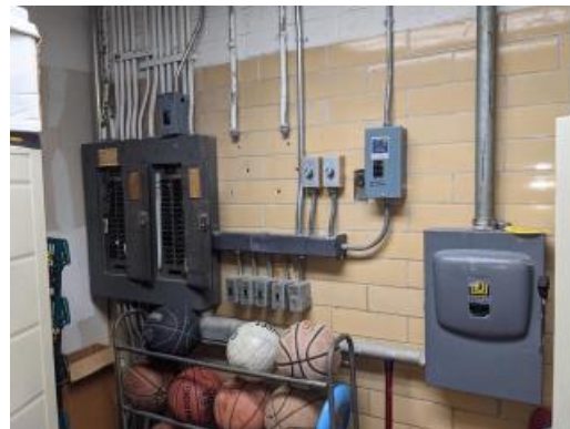
Obstructed electrical panels
