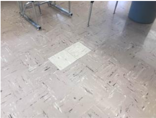
Deficient classroom floors
