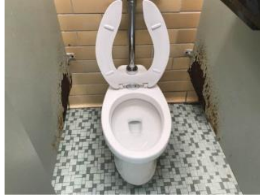
Boys Restroom partitions rusted and beyond service life
