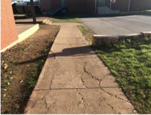
Damaged east side sidewalk
