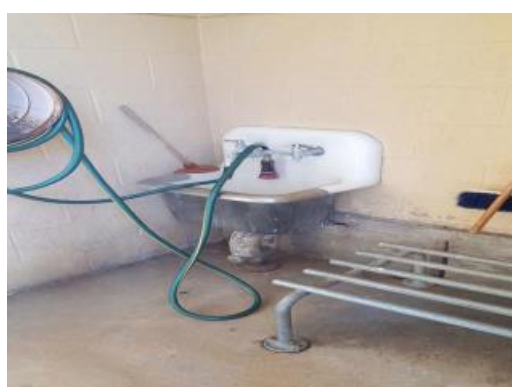
Typical mop sink
