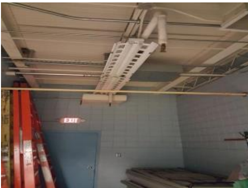
Deficient interior lighting
