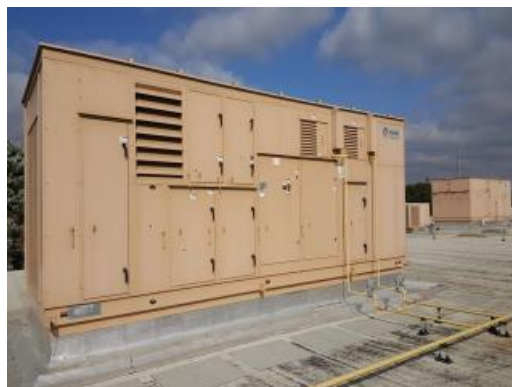
Roof top unit
