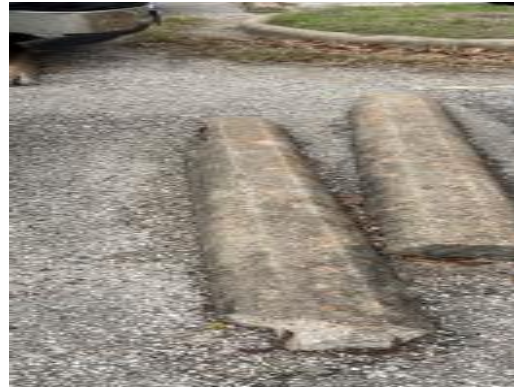
Parking lot concrete stops are damaged or missing
