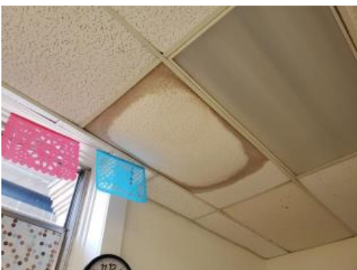
Stained acoustic tiles
