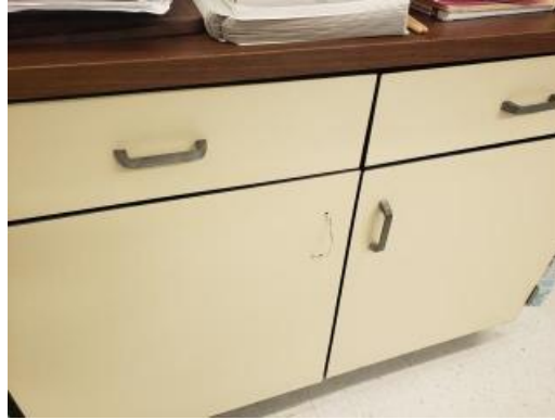
Wooden casework deficient hardware
