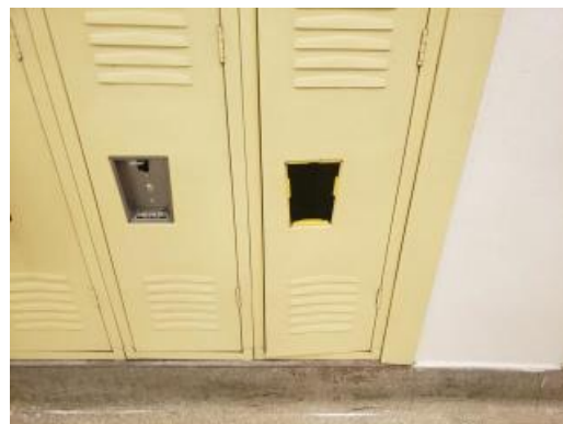
Metal locker deficient
