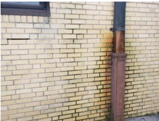
Stained exterior wall
