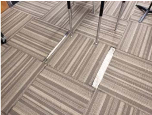
Damaged carpet floor
