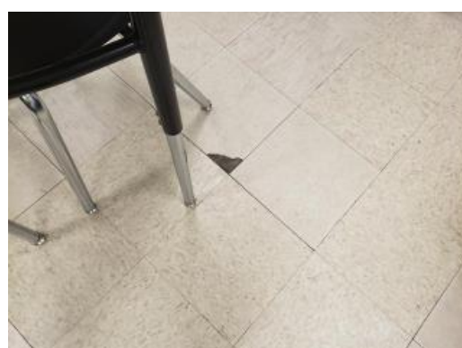
Damaged tile floors
