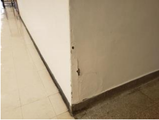
Damaged interior wall
