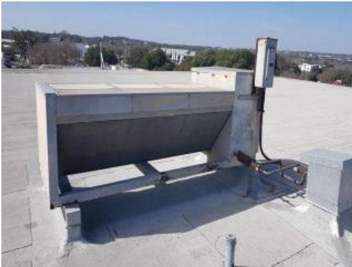
Aged roof top unit
