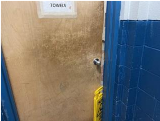
Wood door is well worn
