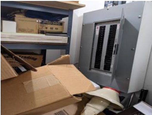
Obstructed electrical panel
