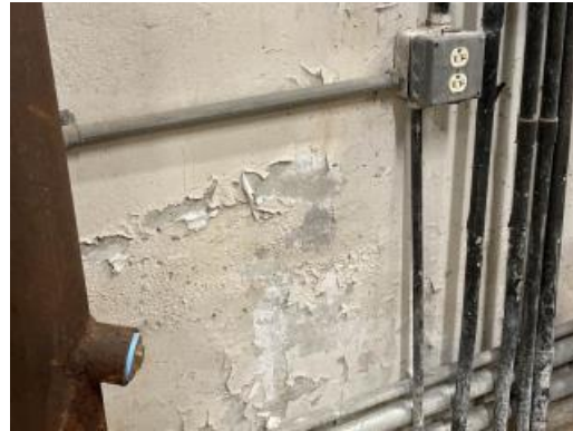
Concrete masonry wall has chipped and peeling paint
