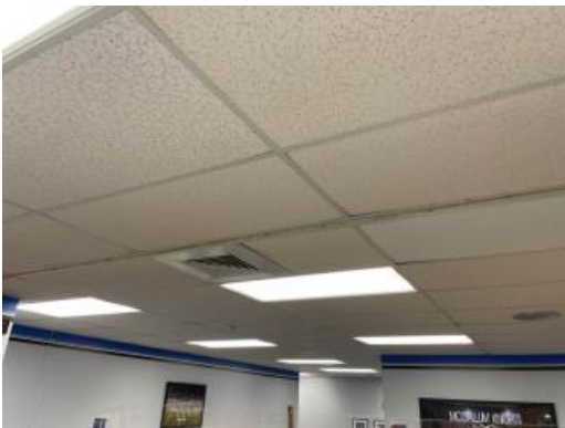
corrosion of acoustic ceiling tile grid
