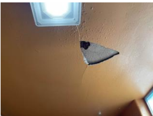
Hole in plaster wall
