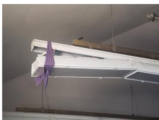
Light fixture is broken
