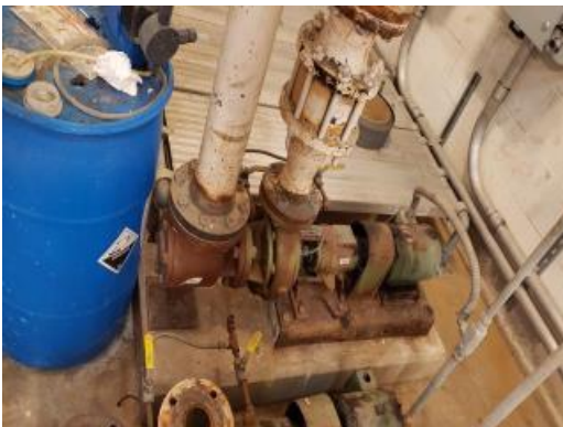
Circulating pump is well worn
