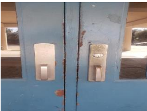
Exterior doors rusted
