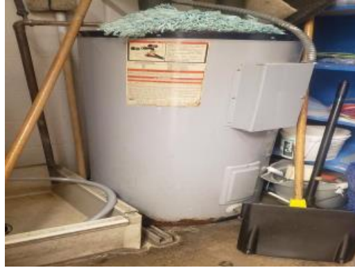
Water heater corroding
