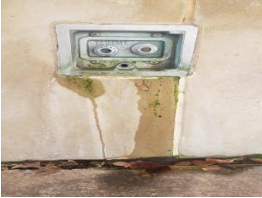
Water spicket leaking
