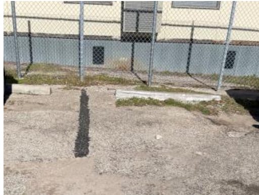
Parking spaces are worn
