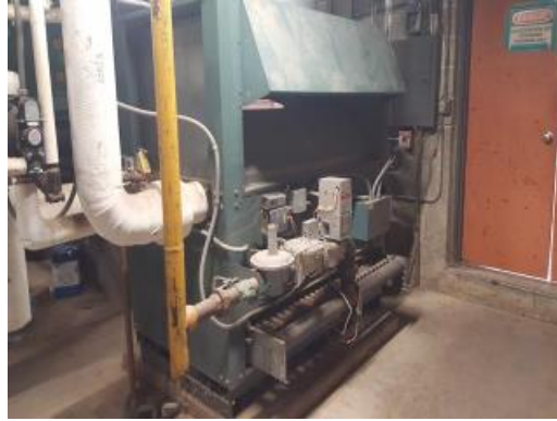
The gas boiler is approaching the end of life.
