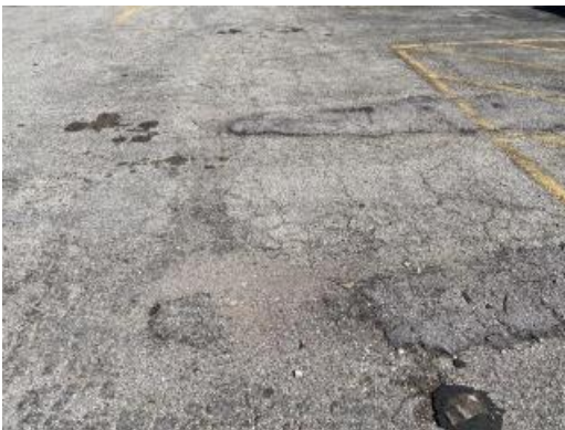
Asphalt pavement needs to be replaced
