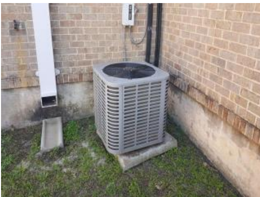
Condenser - looks to be uneven on the concrete slab
