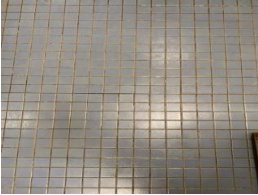
Grout between quarry tiles needs to be redone
