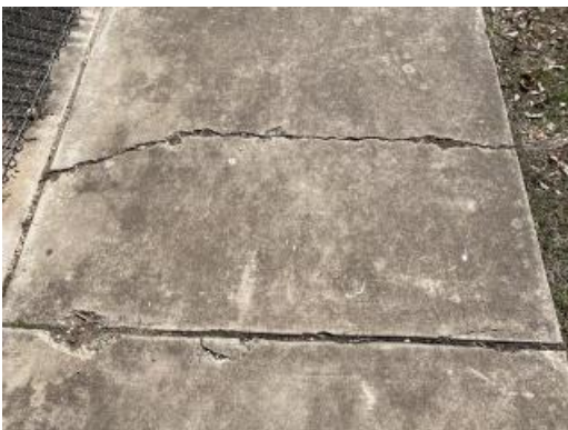
Concrete sidewalks present cracking
