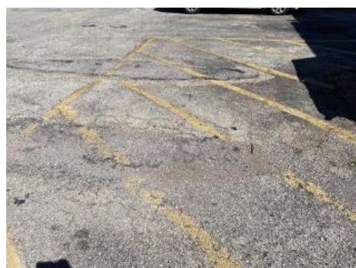
Asphalt needs to be repaved
