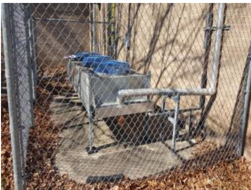
HVAC Condensing unit
