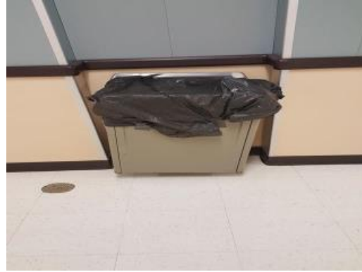
Drinking fountain not working
