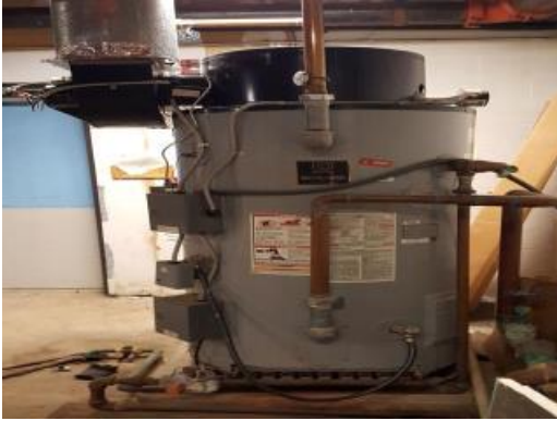
Corroding water heater pipes
