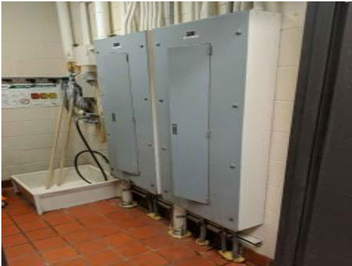
Typical electrical distribution panels
