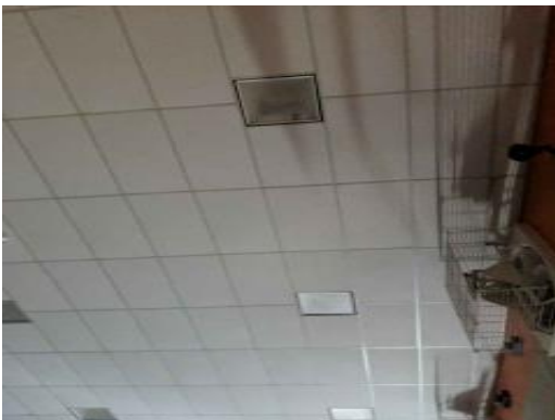
Typical accoustical ceiling
