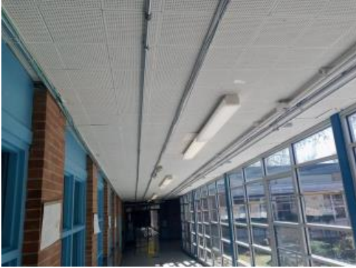
Typical Hallway Finishes
