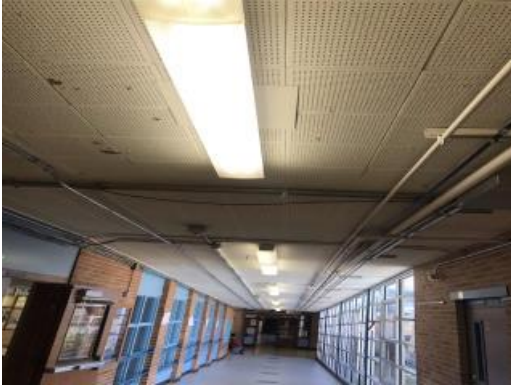
Typical Hallway Finishes
