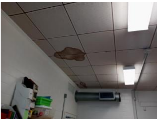
Damaged ceiling tiles
