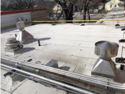
Roof exhausts discolored
