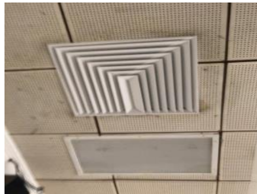
Damaged ceiling tiles
