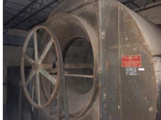
Aged and rusted supply fan
