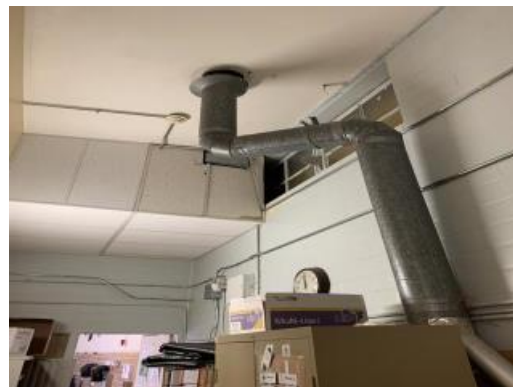
Exhaust is loose from ceiling
