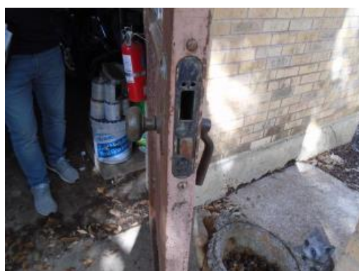
Exterior doors are corroded and beyond their useful life
