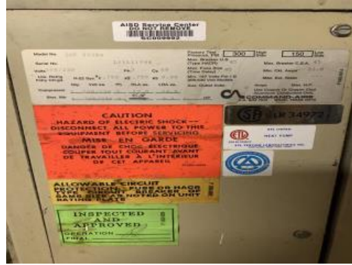
Aged furnace equipment
