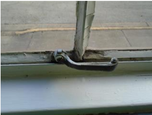
Damaged Window Hardware
