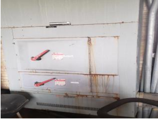
Corroded main disconnect
