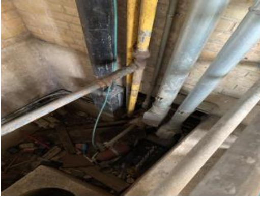
Aged piping systems
