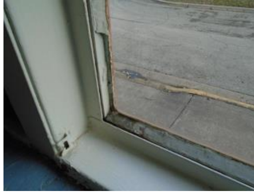
Damaged Window Frame
