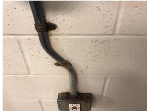
Worn circuit to hand dryer
