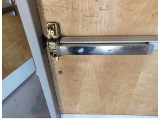
Damaged door hardware
