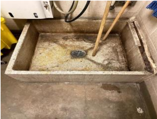
Mop sink heavily used and damaged
