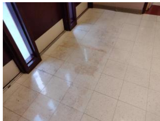
Damaged floor tiles
