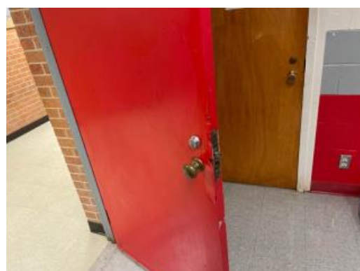
Damaged Interior Door
