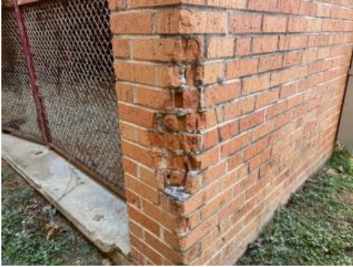
Chipped brick at OLDINC room
