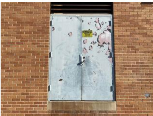
Rusted and paint chipped steel door
