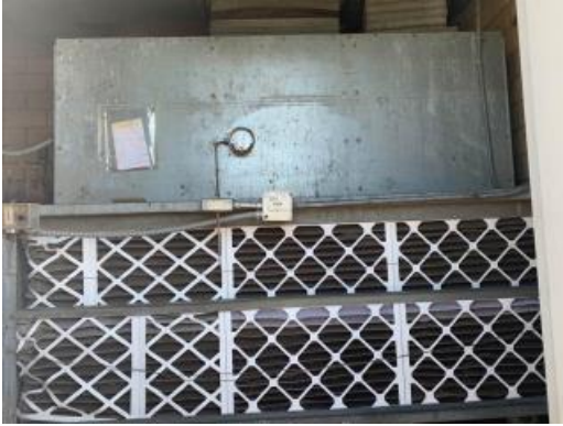
HVAC Unit is beyond its useful life
