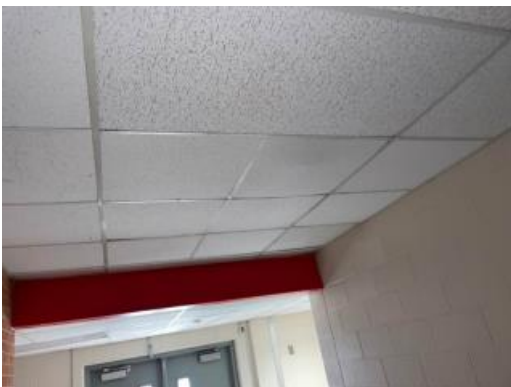
Damaged acoustical ceiling grid and tiles
