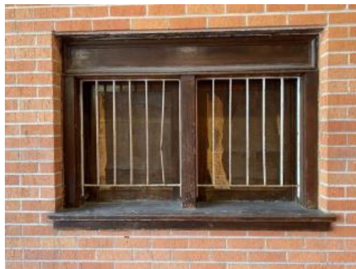
Exterior wood windows are beyond their useful life
