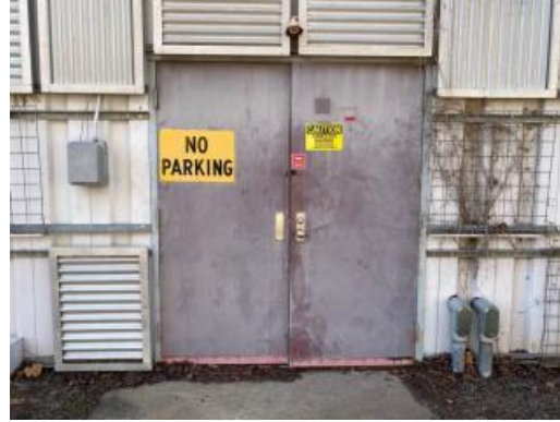
Sun bleached front entry metal doors
