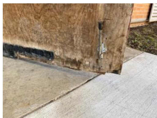
Chipped front wood door
