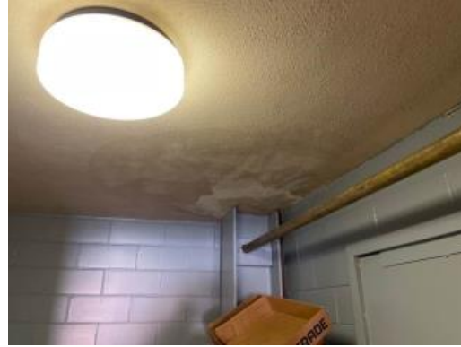
Water stains on ceiling
