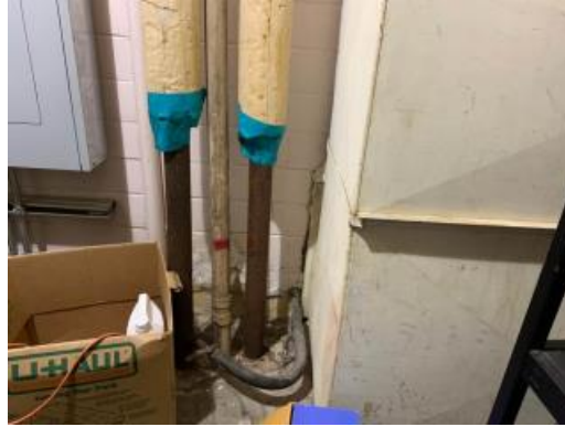
Pipes are showing signs of corrosion
