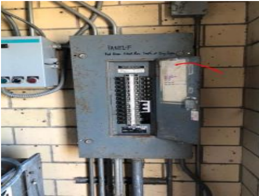
Electrical distribution panel is beyond its useful life.
