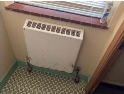
Aged unit ventilator
