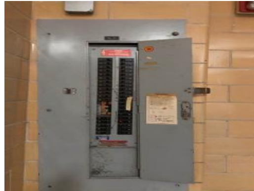
Exposed bus bars
