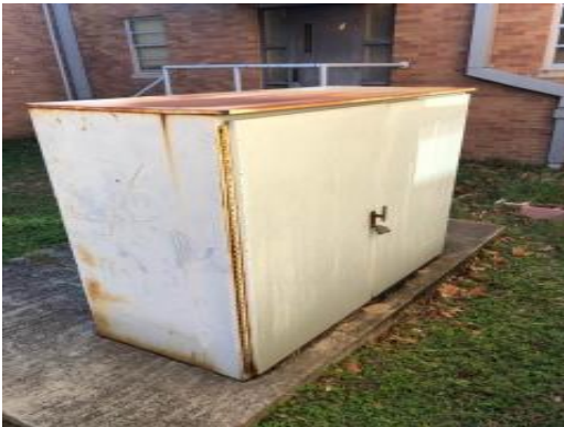
Exterior aged electrical enclosure
