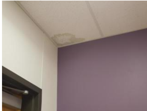
Stained acoustical ceiling tile
