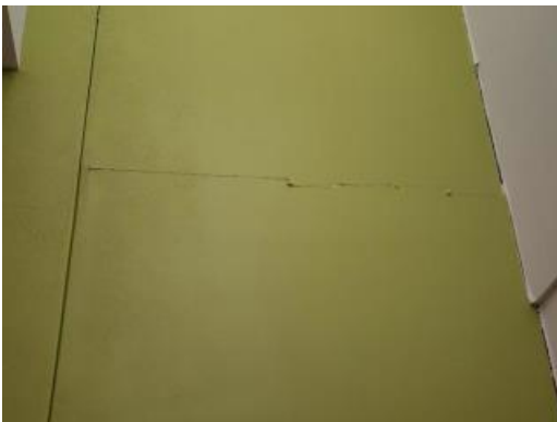
Damaged hard ceiling
