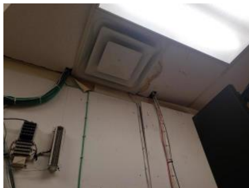
Damaged ceiling diffuser and acoustical ceiling tile
