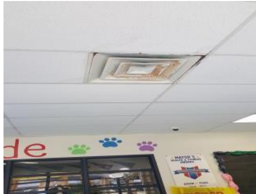
Damaged ceiling diffuser
