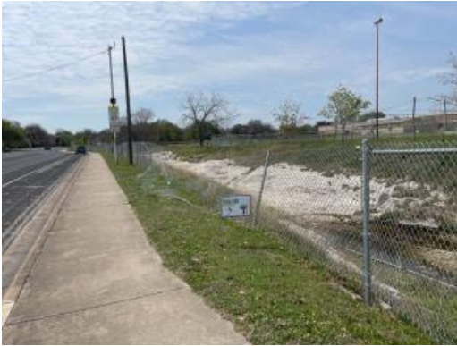
Northeast corner fence damage
