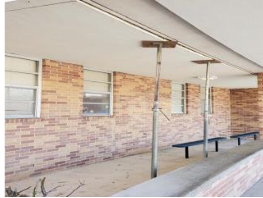
Failing plaster ceiling
