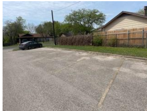
Parking lots need restriping
