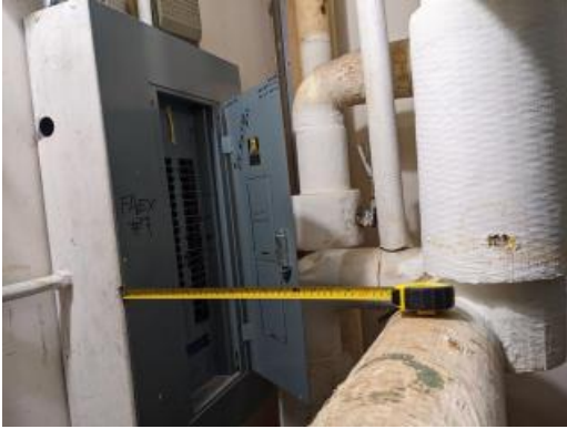
Electrical Breaker is too close to piping
