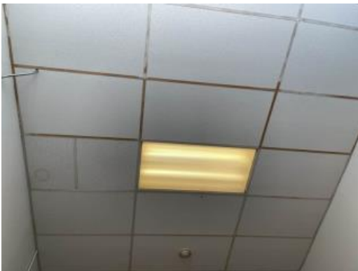
Worn and stained acoustic ceiling grid and tiles
