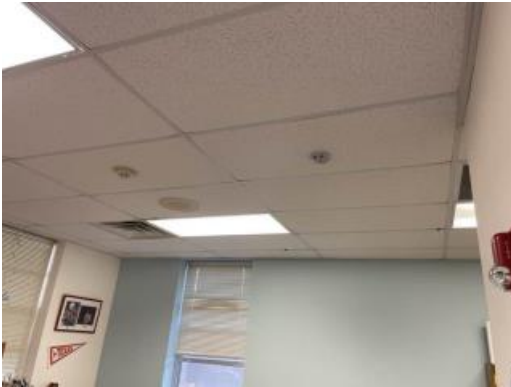
Sagging ceiling grid and tiles in office
