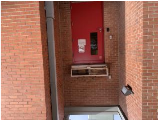
The air curtain is not operating.
