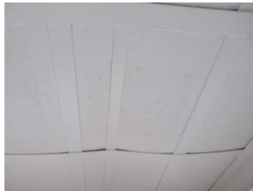
The ceiling grid is bowing and beyond useful life.
