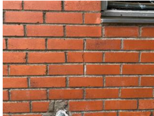
The exterior brick veneer presents cracking.
