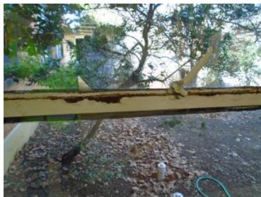
Rusted Window Latch
