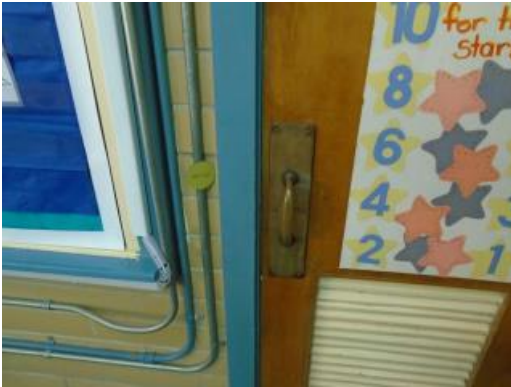
Classroom Doors are dated
