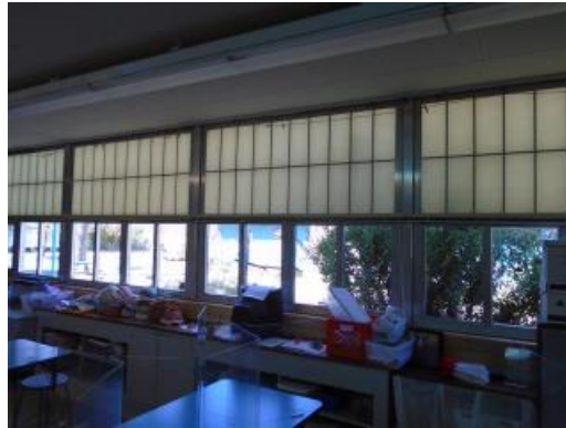
Classroom Windows are beyond their useful life
