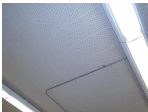
Glued on ceiling is beyond its useful life
