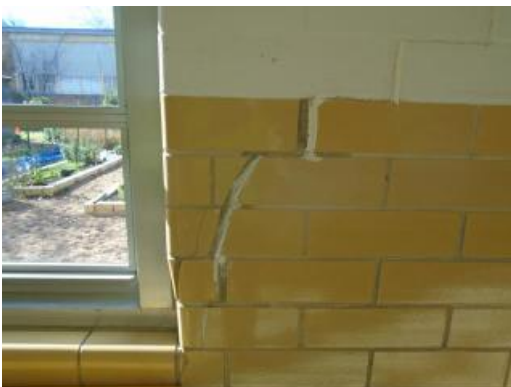
Cracked Brick Wall
